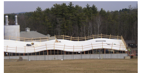
Before the green roof work started, a root resistant waterproofing made by Sika Sarnafil was installed.
