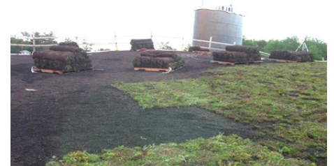
The precultivated vegetation mats were laid butt joints directly onto the green roof substrate.
